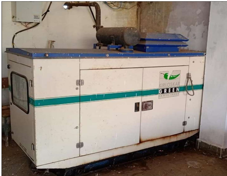
Figure 2.1:- DG set on the college campus
